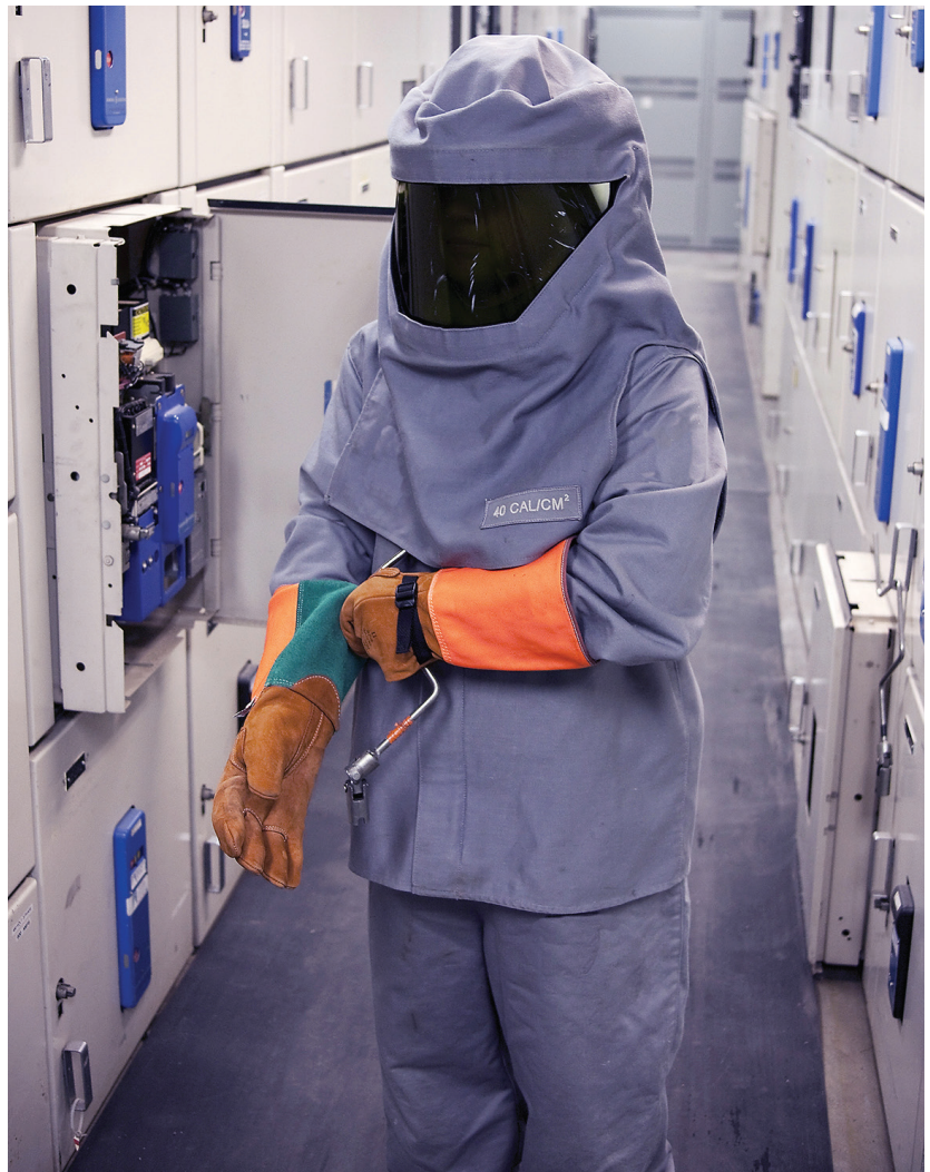
A Cat. 4 arc flash suit protects a technician ready to rack in a low-voltage power circuit breaker.
